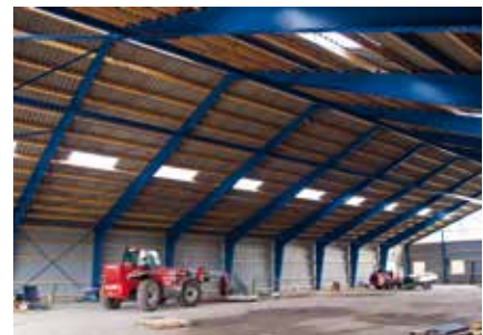
A view from inside the commodious hangar space! Note the twin bracing wires between the steel framework under the roof.
