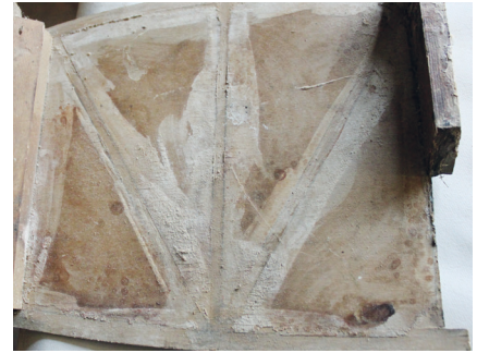
Prototype Kite 1. Stub-spar webbing showing completely failed joints with soldiers removed. Note the 'brown tinged areas' around where the actual joint was originally clamped under pressure. Photo: David Underwood
