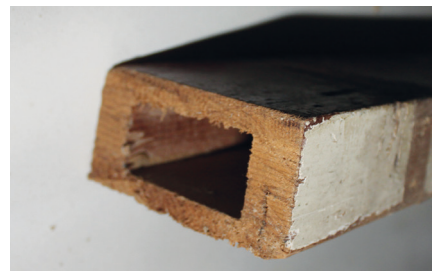
An example of good longevity. Note the soundness of the joints in this 1917 Bristol F2b box-spar. Photo: David Underwood
