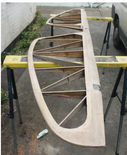
The original elevators were in pretty good shape requiring only relatively minor repairs. Photo: David Underwood
