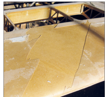
Extent of the delamination of some of the leading edge plywood.
