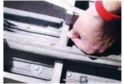
Closer inspection can often highlight glue failure.
