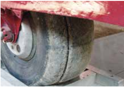
Tyre's will invariably need close inspection. Rubber hardens and cracks with time.
