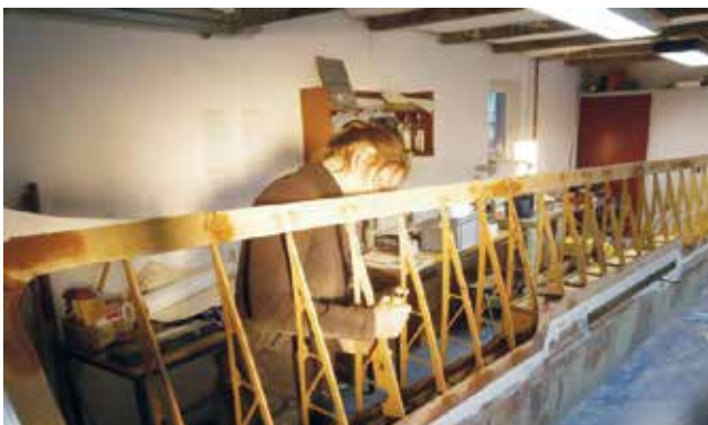
Some of the rib-gussets were damaged and required careful removal with sharp tool.
