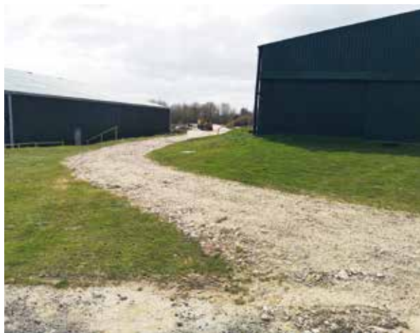
A new access road for the new workshop has been constructed between the hangars. (Gary and Richard's skills could surely be of valuable assistance in rebuilding some of the nation's sorely lacking B-roads!).
