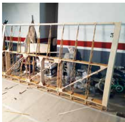
Work on an SG-38 in Madrid progresses with one wing now completed. Coronavirus confinement will hopefully see things speeding up towards its successful completion? Photo: Carlos Bravo
