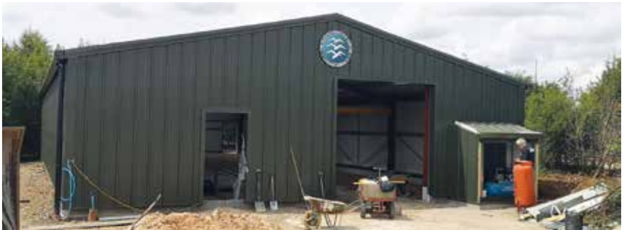
The Welsh contractors certainly didn't let corona dampen their spirits! A complete shell of probably one of the most important buildings at the GHC. What's next Mr Pullen? Photo: Paul Haliday
