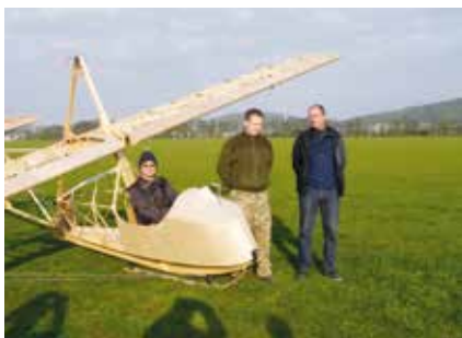
The SG-38 under construction at the Hranice aeroclub. From left to right, the late Pavel Hrinik (seated), Martin Skařupa, and Radek Sohr.
