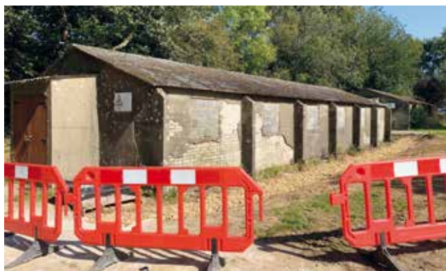
The building before work started. The outside will be next year's painting project.
