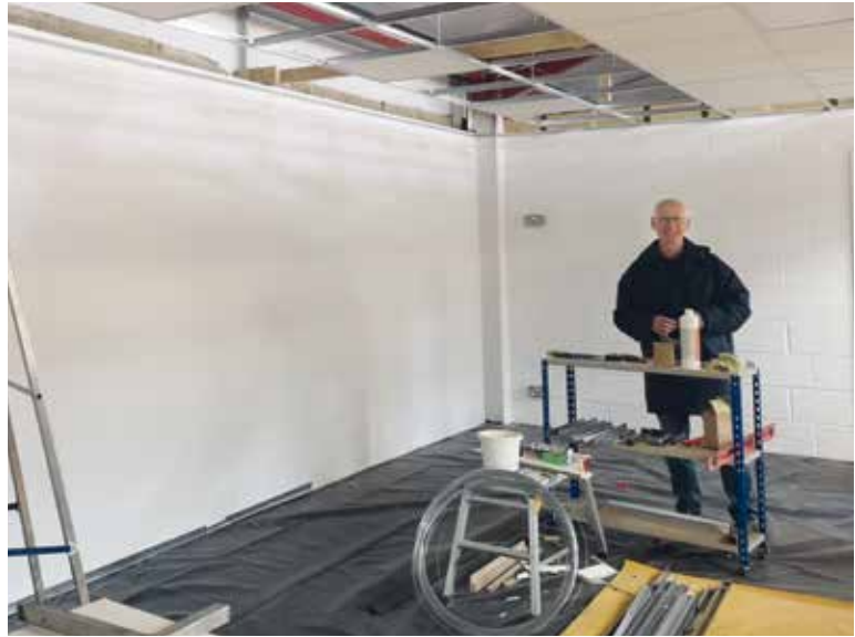
David Siddell turned out to be one of the dark horses that kept everyone in 'suspense' as he installs the suspended ceiling in the machinery workshop. Photo: Paul Haliday
