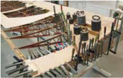
Nearly ran out of glue clamps there! More new structure going into the Lemelerveld T21, with work expected to take another two years. Photo Eric Munk
